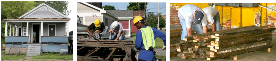
319 Marcellus Street (front), hands-on deconstruction training at 319 Marcellus, timber from 319 Marcellus Street salvaged for a new garage on the same site.
